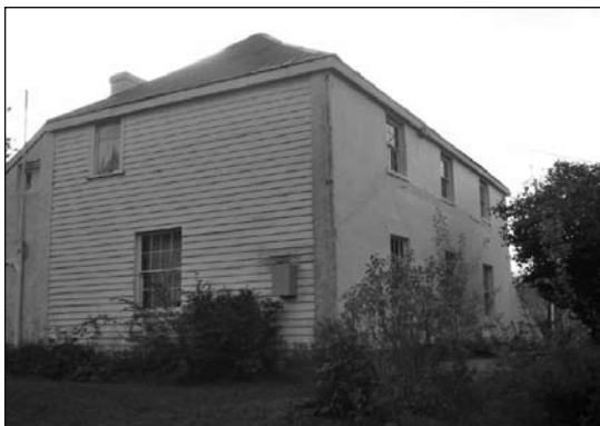
Riversdale Mill on top and house during renovation work. This picture shows nothing of the beauty but much of the size of the task.
