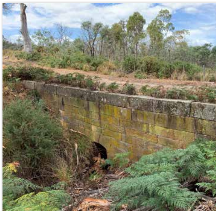
Figure 4. A sandstone culvert on the convict road, just behind Woodsden homestead. Photograph by Malcolm Ward
